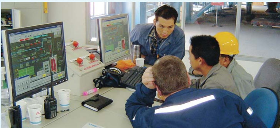
The ISASMELT control room at CYMG featuring MIPAC-designed and configured control interfaces.
